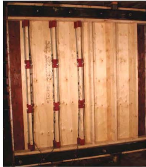
(b) Strengthened wall (left) and as-built wall (right) prior to shock tube testing
